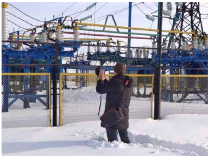
Image 1: Partial discharges need to be located from a safe distance.
